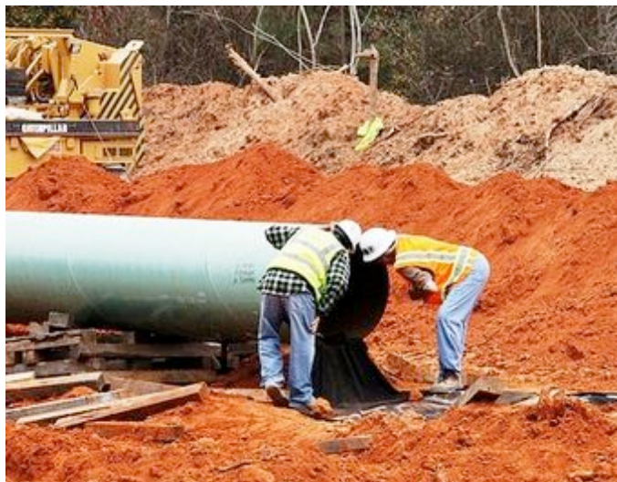
Workers examine pipe being used for the southern leg of the Keystone XL pipeline. Credit: Steven DaSilva, Fredonia Rebel Post, flickr
