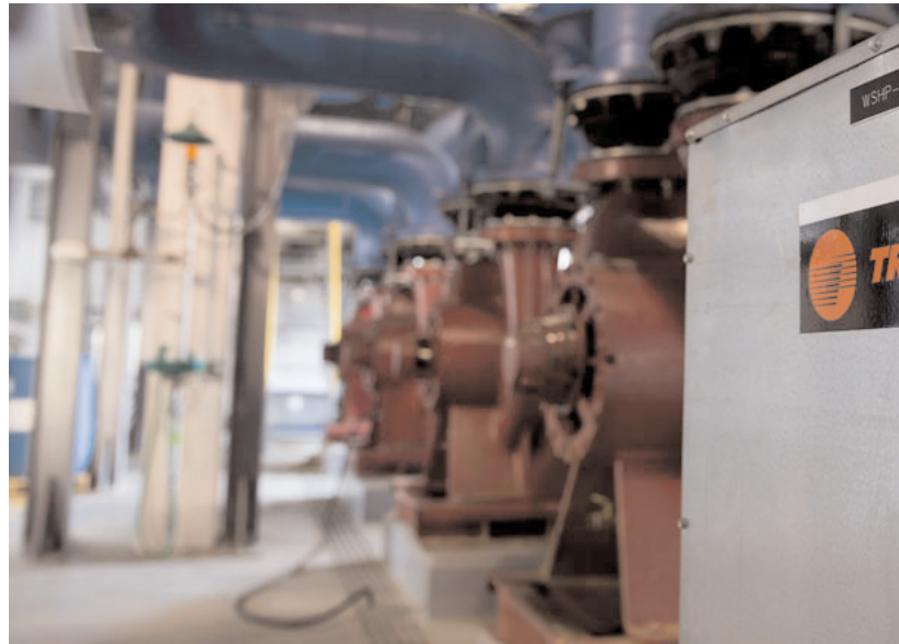
This heat exchanger plant at Naval Air Station Oceana's Dam Neck Annex in Virginia Beach, Virginia was built by Trane, a subsidiary of Ingersoll-Rand Plc. Photographer: Andrew Harrer/Bloomberg
